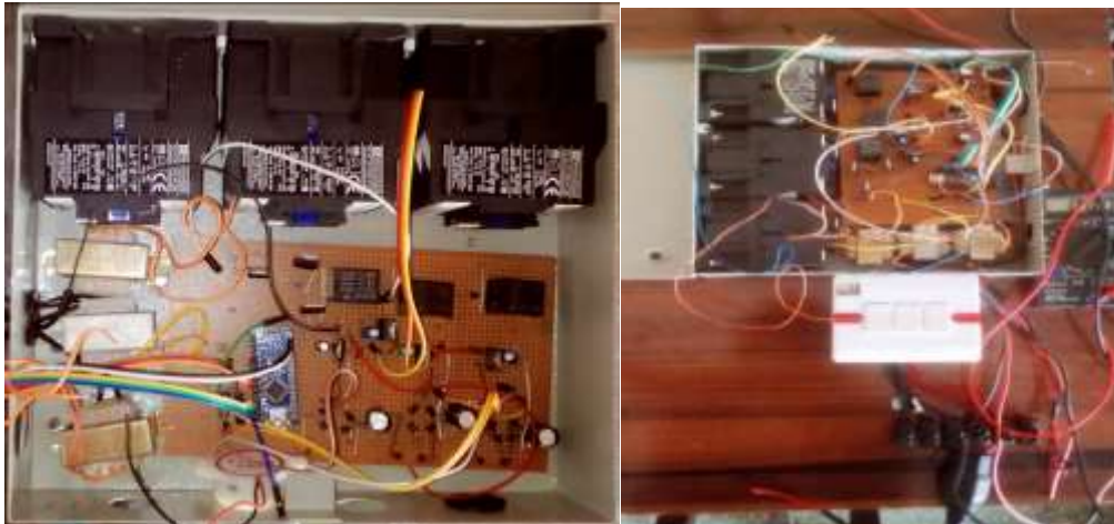
Figure 9: Arduino-based 5kva Automatic Power Transfer System
