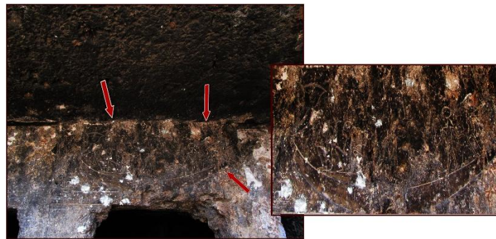
Figure 2: Change of color; one of the most common deterioration patterns of fire damage in the North Chapel
