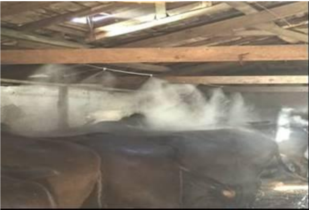
Figure 2: Barn-I, where the fogging system was installed
