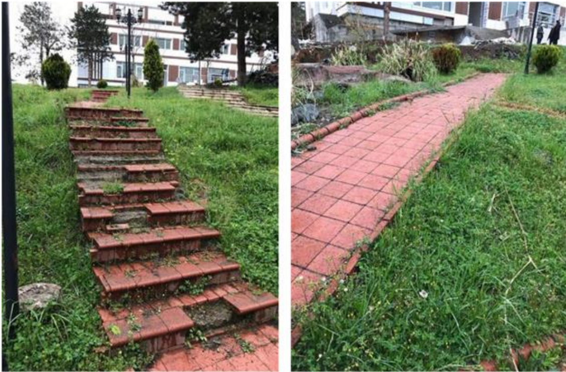
Figure 6: Examples of existing roads that are usable and need to be renovated
