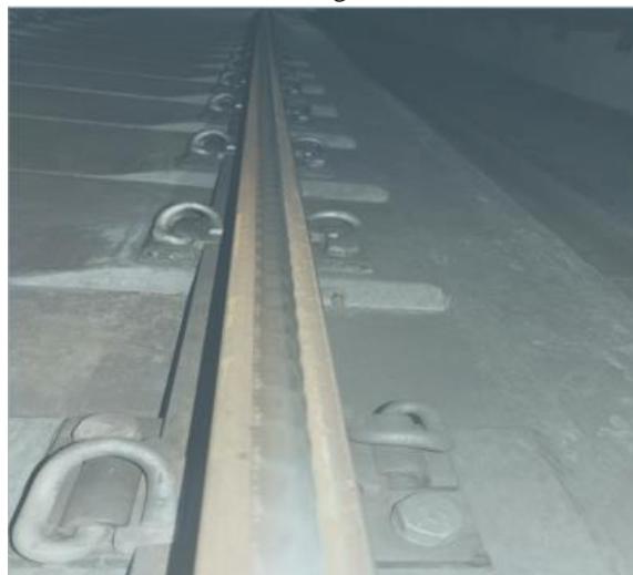
Figure 3: More severe wave wear rail
