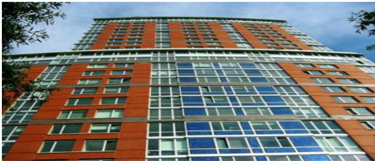
Figure 3: Building façade with integrated photovoltaic panels [9]
