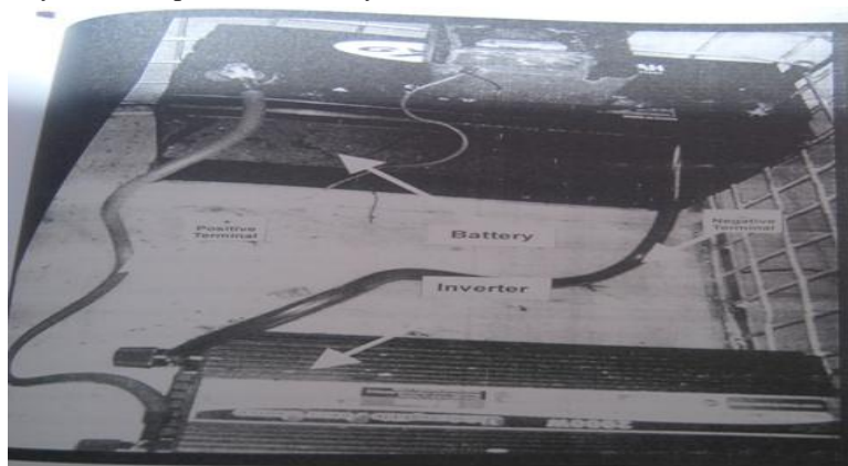
Figure 6: The Assembly of the Inverter and Battery
