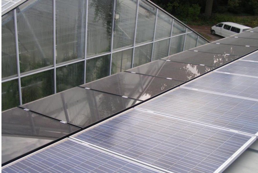
Figure 3: Solar panels on top of the visitor's center
